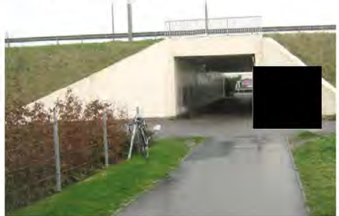
Figure: 10.52 Underbridge (cycle and pedestrian-only) with divided carriageway above to create opening – Lund, Sweden
