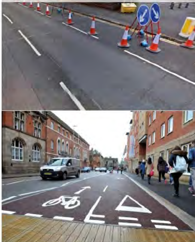
Figure 6.2: Newark Street, Leicester – Trial of traffic lane closure and new two-way cycle track taking the place of the coned-off lane
